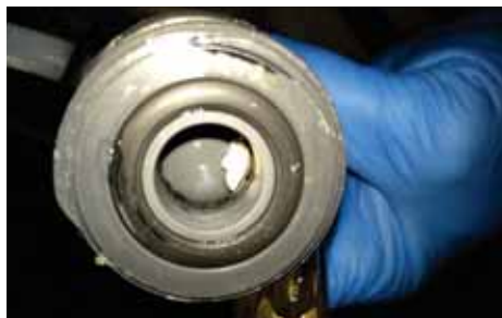
check valve scale buildup examples
